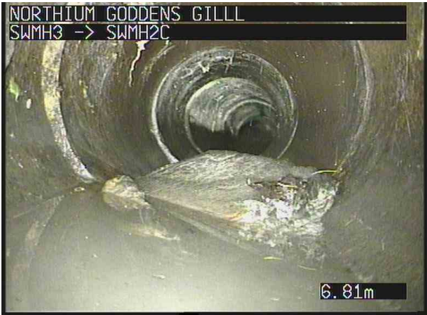
Sec_4_Insp_1_SWMH3X_35791.jpg, 00:00:54, 6.81 m Settled deposits, hard or compacted, 20% cross-sectional area loss
