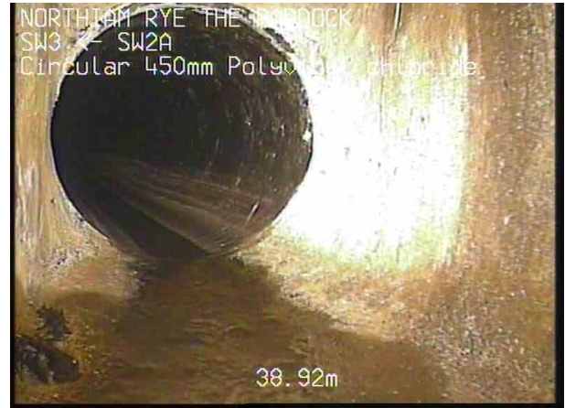
SW3_U_220225_103840__6.jpg, 00:03:31, 38.91 m Finish node, manhole, reference: SWMH2B, Screen Text should read SWMH2B not SW3
