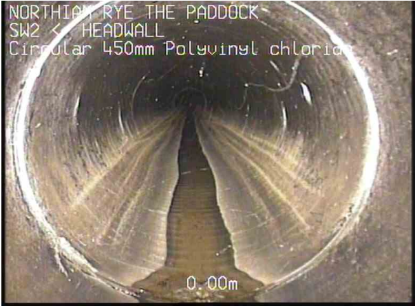
SW2_U_220225_095819__1.jpg, 00:00:00, 0.00 m Start node type, other special chamber, reference number: HEADWALL, HEADWALL
